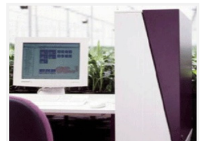
Integrated systems control
